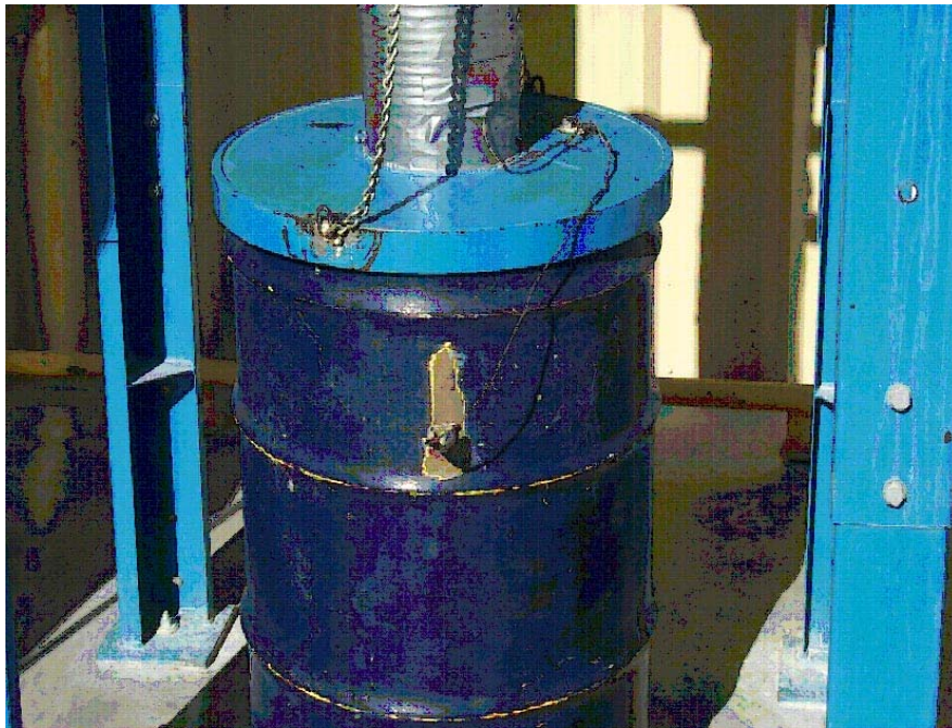
Figure 2 Dust collection drum grounded to flexible duct. (courtesy Gowan Milling, LLC)
